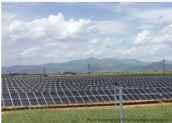
Photo Courtesy by TESCO Engineering/Inergion
